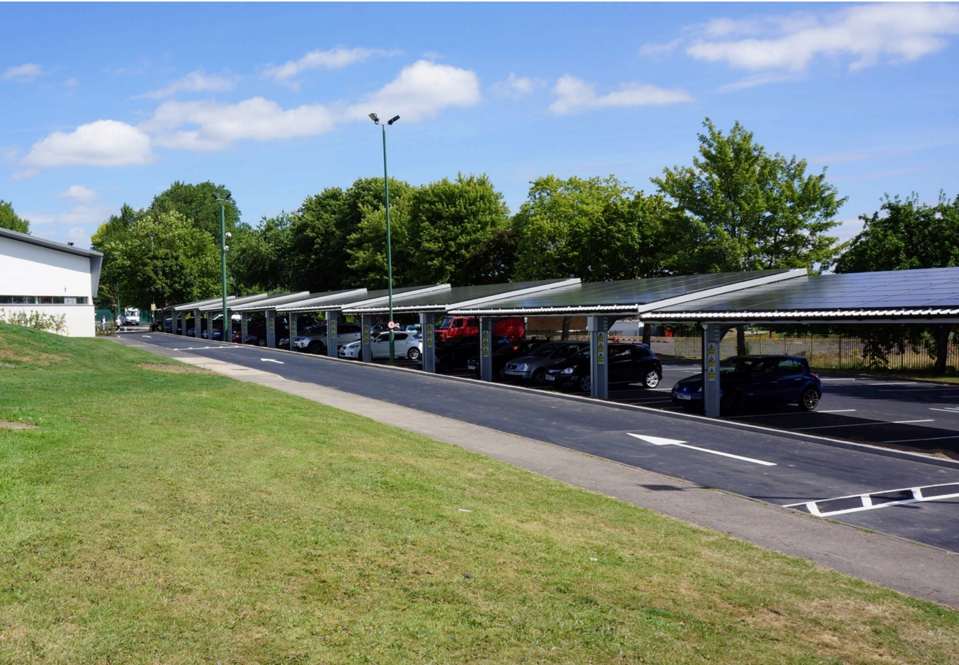
Flexisolar PV/EV System - Nottingham, UK
